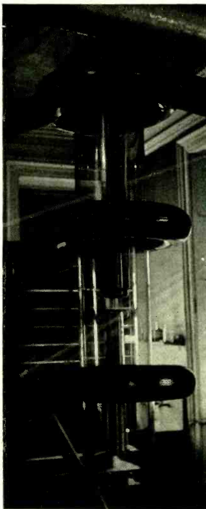
Rectifier tower at New York University, showing string controls in foreground and stove pipe wiring.
